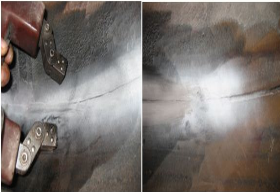
Figure 1. Crack observed in the connections root
