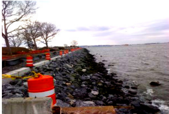
Photograph 3: Seawall conversion from wall to revetment moves the shore 15-feet landward and provides more protection to the shore line by dissipating the energy on the most active side of the island over the incline of rip-rap stone (photo facing southwest).
