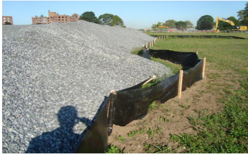
Photograph 2: PPS-I silt fence surrounding several lifts of general fill – never experiencing sediment migration
